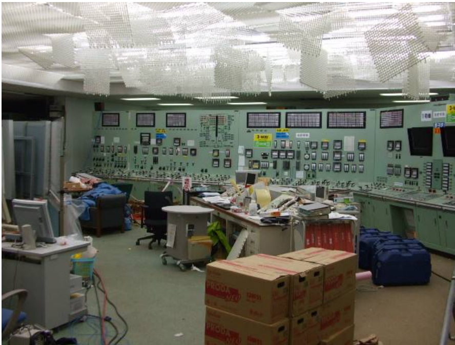
Unit 1 Main Control Room lights turned on (The light covers come off by the earthquake)
