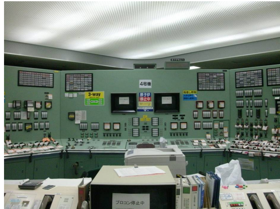
Unit 4 Main Control lights turned on
